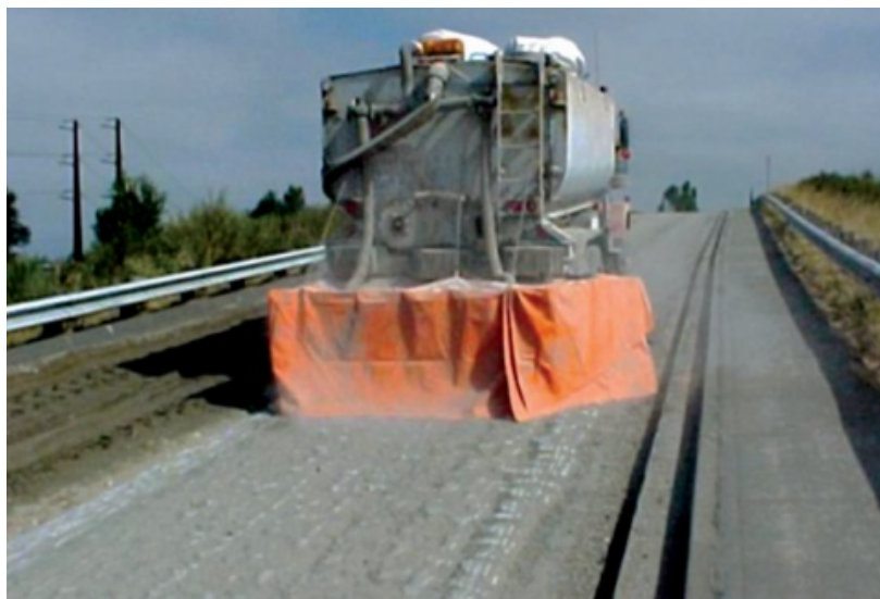
Figure 2. In mixed-in-place construction, cement is uniformly distributed over the area to be processed
